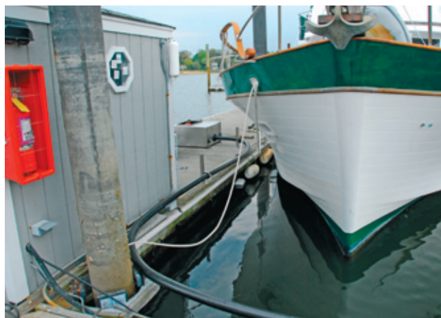
Connection to the dispenser sump
